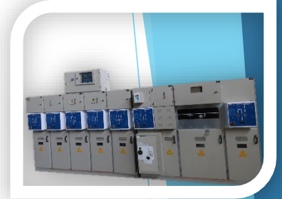
Compact Metal Enclosed Switchgear
